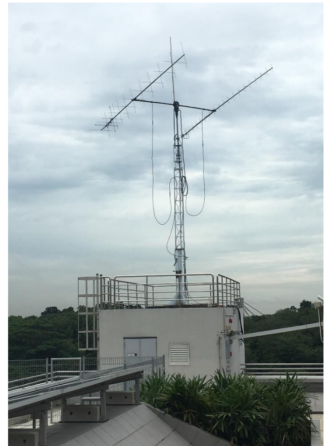
Ground Station: Located in NTU
